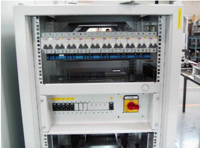
Distribution line with 2P breakers
